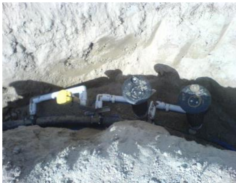
Figure 11. QCV and greens 'back to back' sprinklers.
